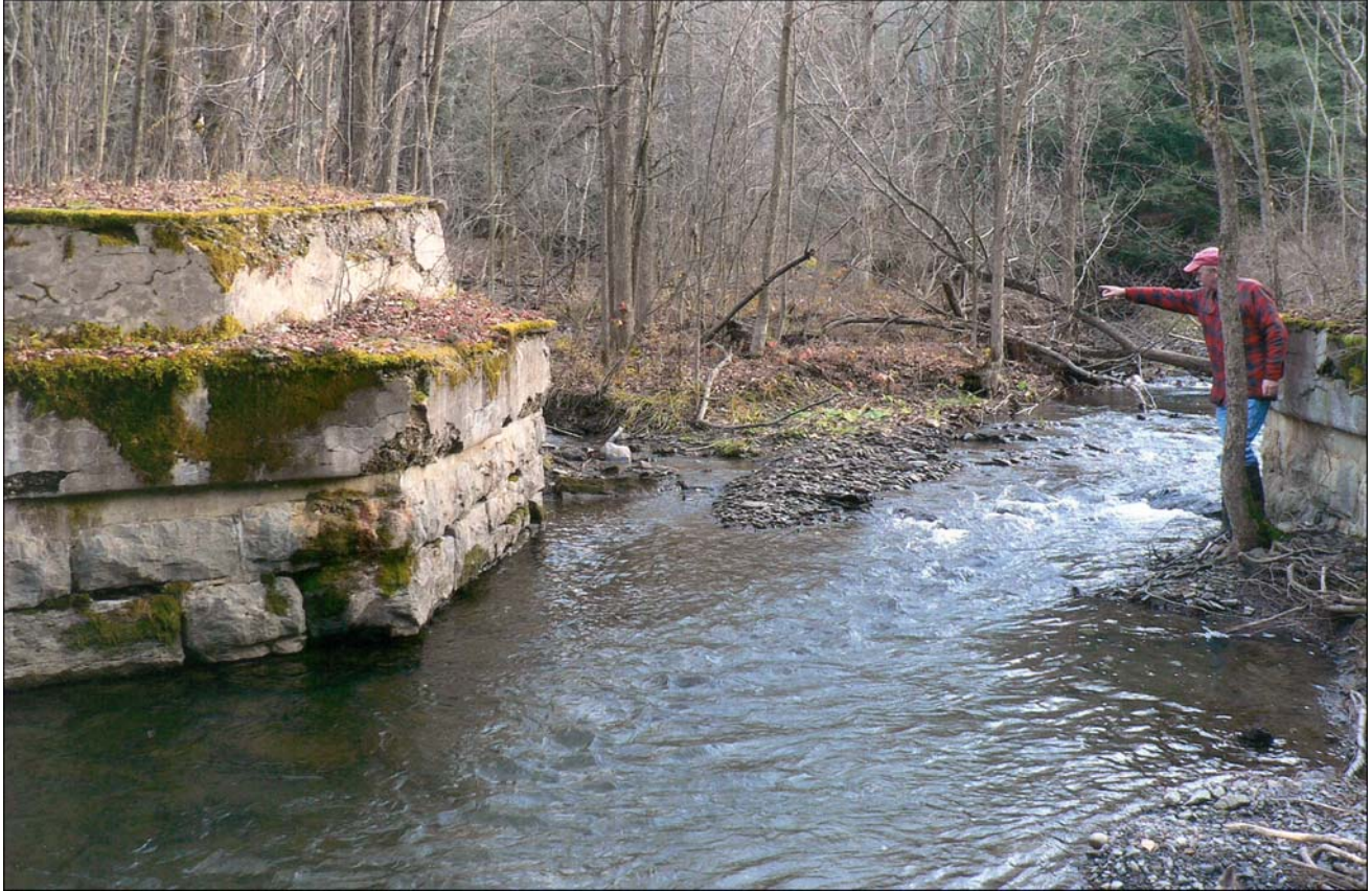
Besides the Chenango's tunnel and five of its stations, many of the line's bridge abutments also survive. In this scene, above, Jim Georges points to the remaining stonework for bridge E-46 with Georgetown Creek still coursing between the abutments. Photograph by Janice Georges.
